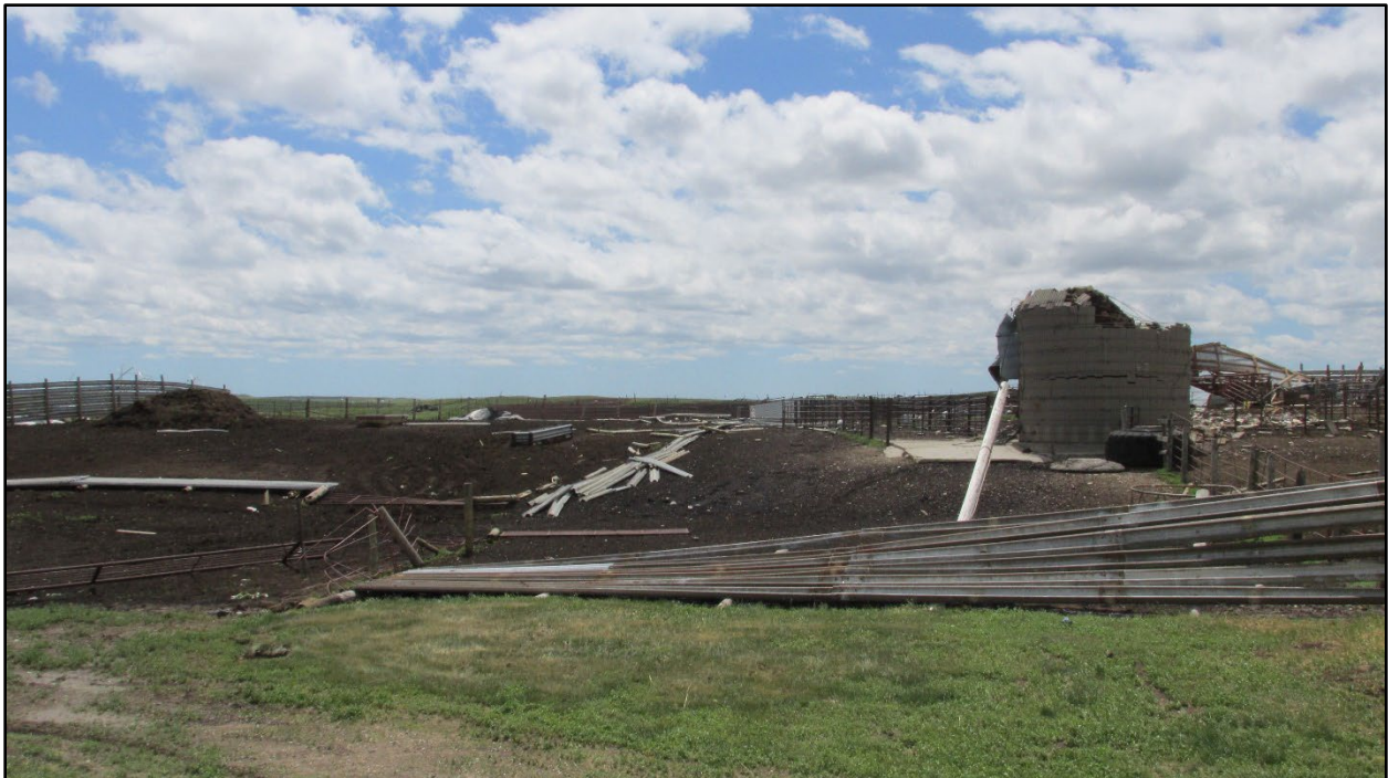
Figure 4.11.5 – June 22, 2016, Severe Storm Damage in Logan County, North Dakota
