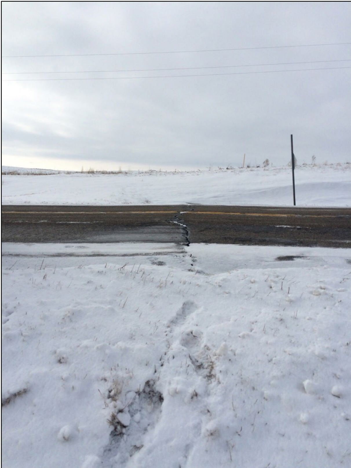
Figure 4.8.3 – 2017 N.D. Highway 46 Frost Heave East of the City of Gackle
